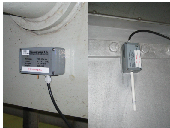
Figure 3.20. Pressure sensor (left) and temperature and humidity sensor at turbo charger (right) for engine room conditions.
