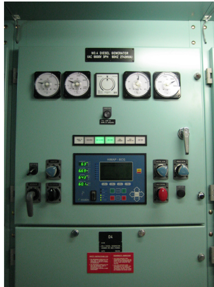
Figure 3.22. Generator control switch board.
